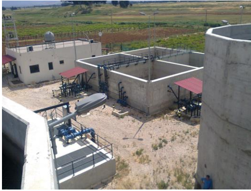
Ablah, Lebanon – Waste Water Treatment Plant
